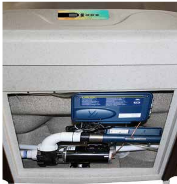
Equipment access is below the topside control panel on most spas.
